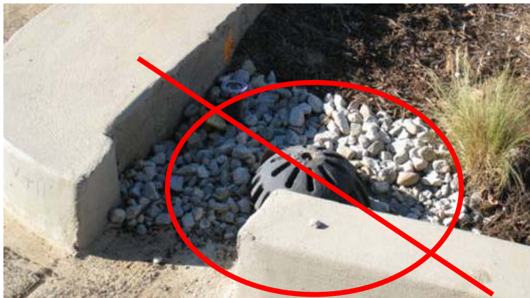
Figure 6: Incorrect Placement of an Overflow Inlet.
