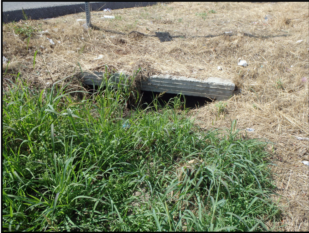
PHOTOGRAPH 1 - The onsite, ephemeral drainage feature (D1) is fed from a storm drain outlet at the northwest corner of the Project Site and flows south.
