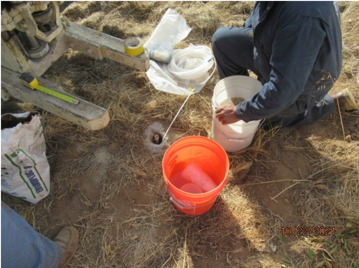
Photo 2 - Soil vapor probe construction at location SVP-5 is shown. The deeper 10-foot soil vapor probe is already installed with the 5-foot probe due to be installed utilizing the plastic pipe shown in the borehole next to the 10-foot soil vapor probe tubing. Construction materials include sand, bentonite granules, water, plastic tubing, and plastic probe tip inserts.
