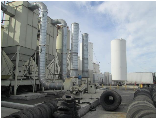
13. Liquid nitrogen tank (background) and dust collection systems (left).
